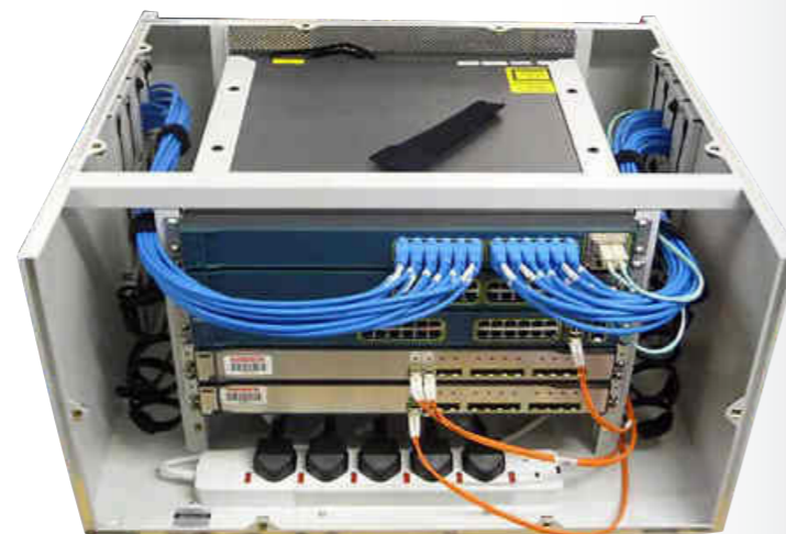
Complex cabling and harness management can be designed in to suit customers' specifications
